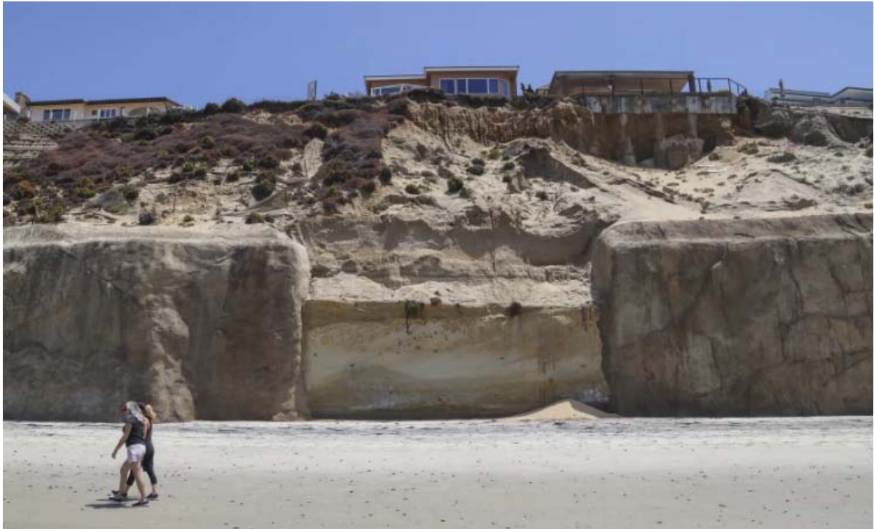
The California Coastal Commission approved a seawall Thursday to fill this gap at 245 Pacific Ave. in Solana Beach. (Eduardo Contreras/The San Diego Union-Tribune)
