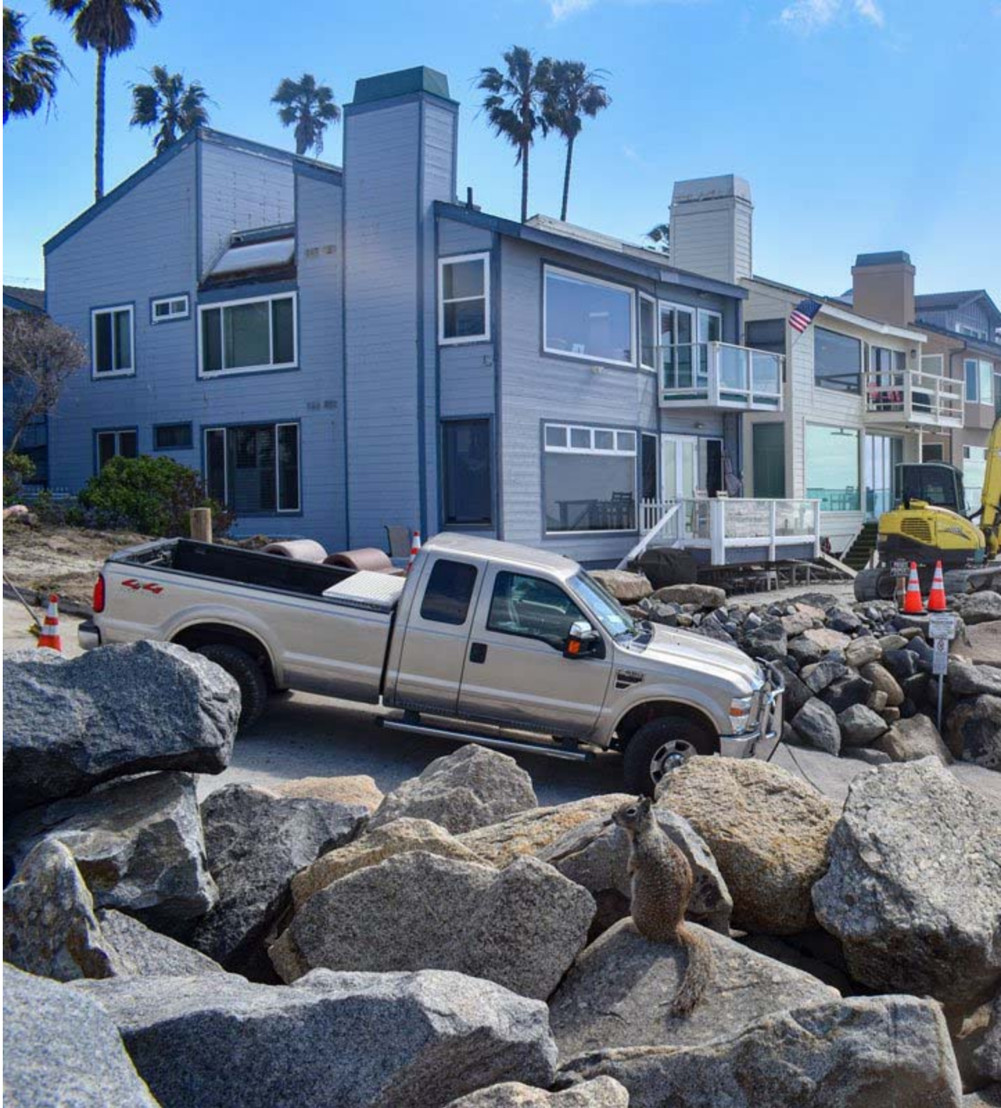
The city said the work was to repair damage made to the revetment from a recent storm while local activists argue that the property owners are taking more public beach access away for themselves. Photo by Samantha Nelson
